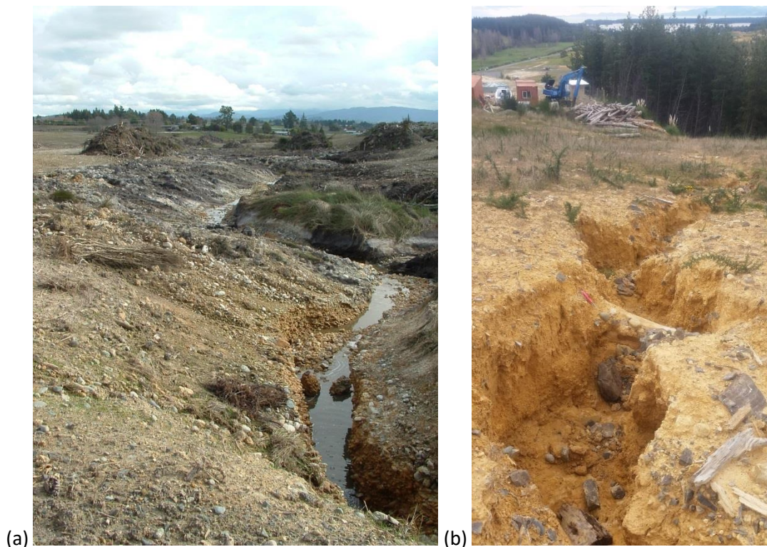
Figure 13: Sediment runoff from (a) site of cleared forestry/recontouring, and (b) Boomerang Farm subdivision
