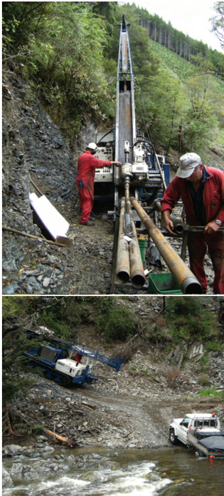
Figure 2: Fording the river and drilling to check dam foundation conditions and carry out water pressure testing
