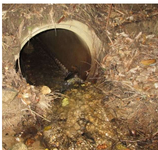
Inlet of Awaroa Rd Culvert 9, Jan 2014. Mussel spat ropes on the inside of the pipe slow down the water to allow better fish passage.
