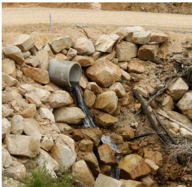
Totaranui Rd Culvert 31 with rubber apron and mussel spat rope attached to the outlet to encourage fish passage (Dec 2012).
