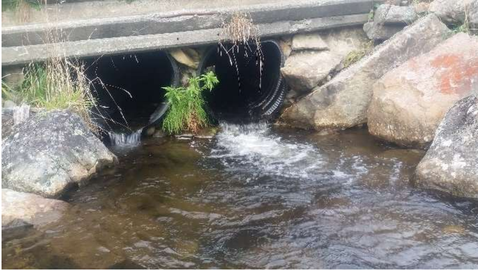
Roundell Creek at Tophouse, showing perched culvert outlet (creating a short waterfall and potential barrier to fish passage).
