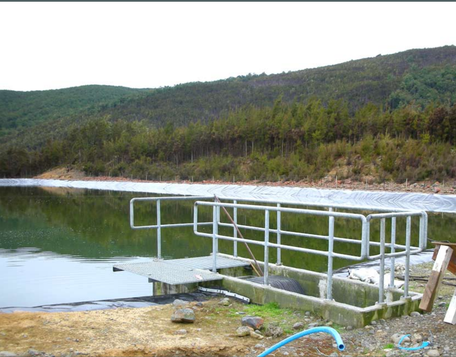
St Arnaud wastewater treatment plant
