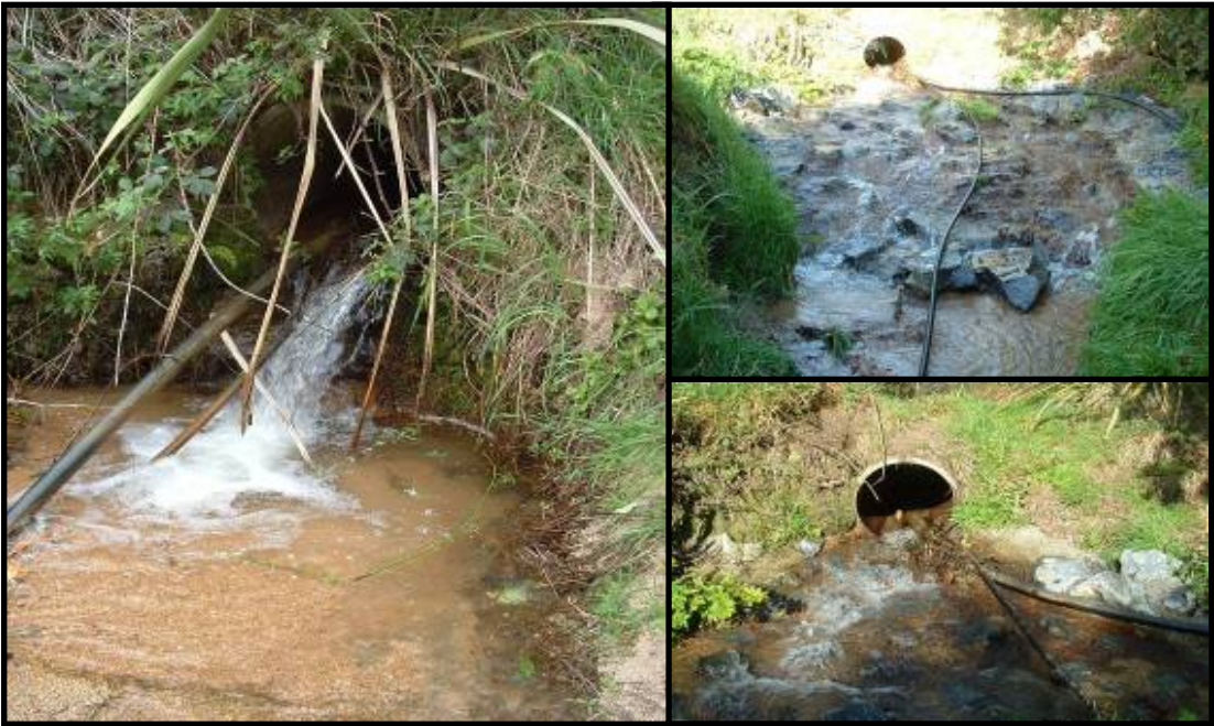
Figure 105: McShane Rd, Wainui Bay (Culvert 9) on before (left) and after remediation for fish passage
