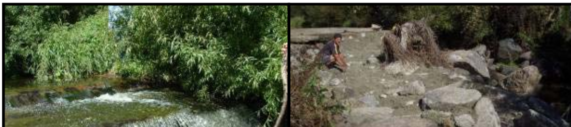
Figure 103: Conveyor belt material bolted on to the outlet end of culverts to assist fish passage
