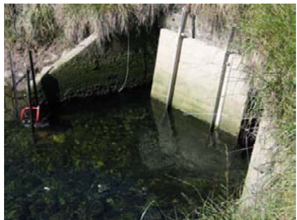
Figure 98: Tidal flap gate at Pearl Creek.
