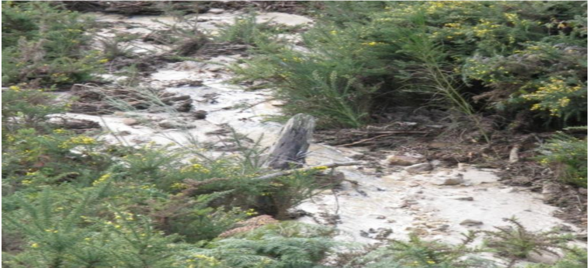
Erosion from poor sediment and erosion controls in road construction in granite geology.
