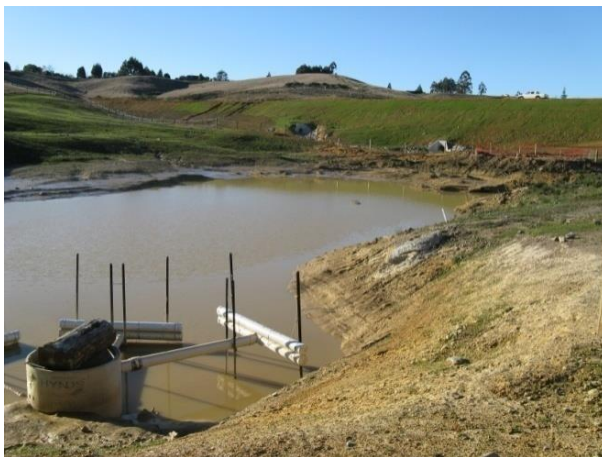
A sediment pond with decanter, Ruby Bay Bypass Gardner Valley Catchment, Moutere.
