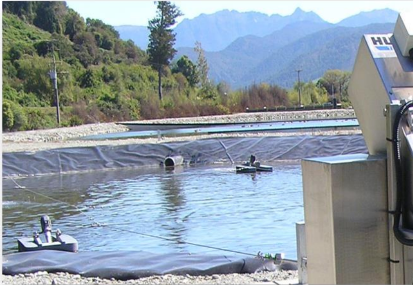
Murchison Sewage Treatment Plant.
