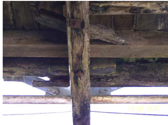
Photo 4: Timber structures are subject to age-related deterioration and may require closer monitoring.
