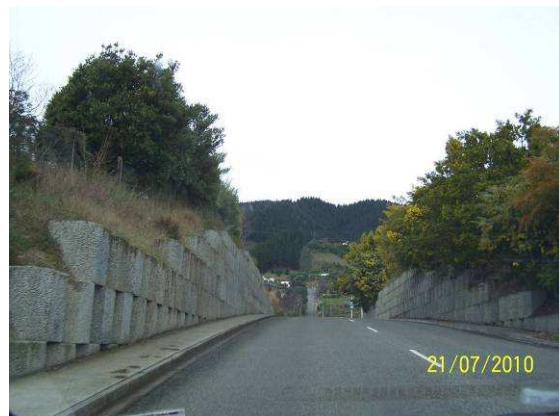
Photo 2: All Structures, including retaining walls, need to be included in regular structural inspections
