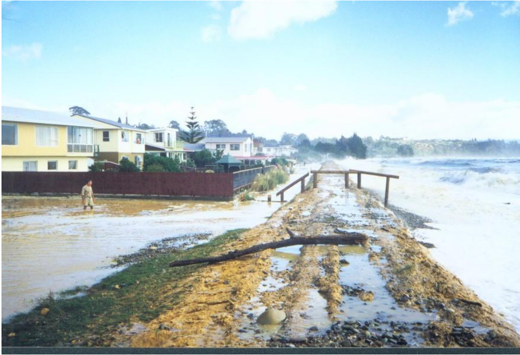
Photograph 2 - Overtopping of constructed clay bank during Cyclone Drena
