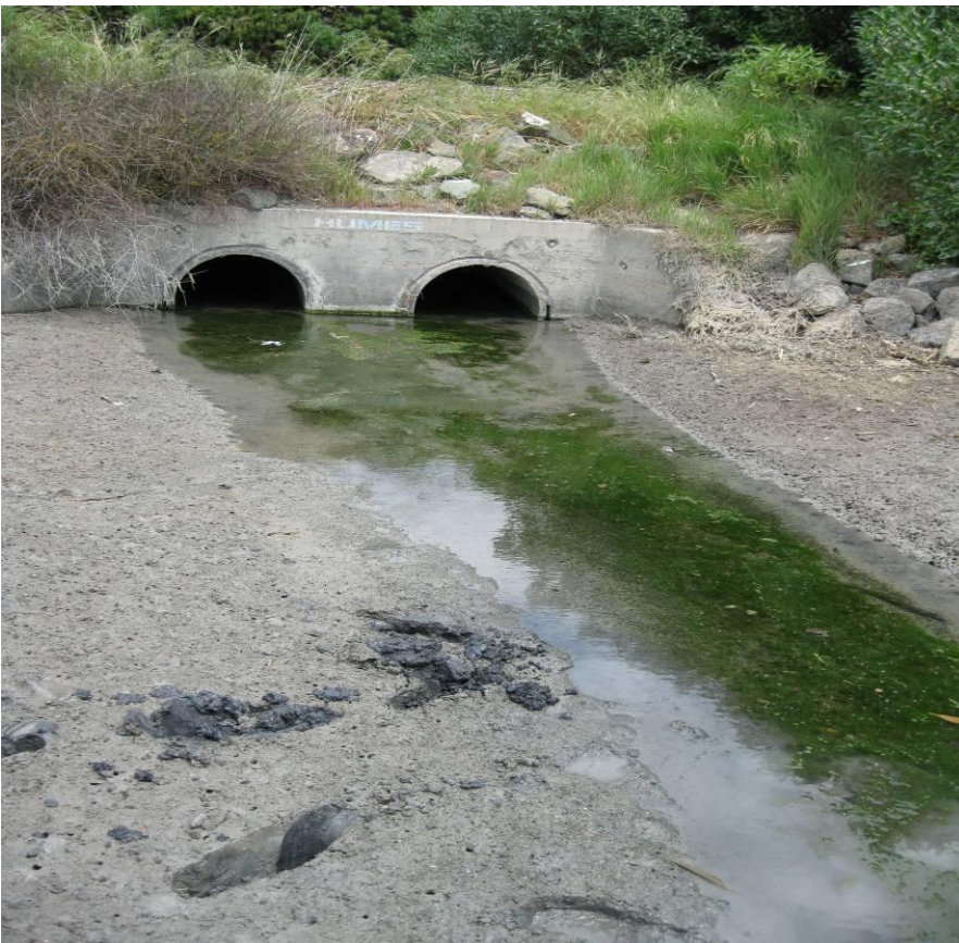
Soft mud at Dynea culvert sample site
