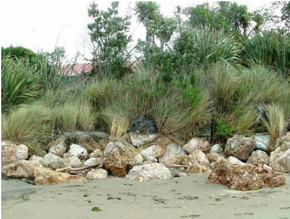
Photograph 4: Photograph illustrating the condition of much of the existing rock revetment
