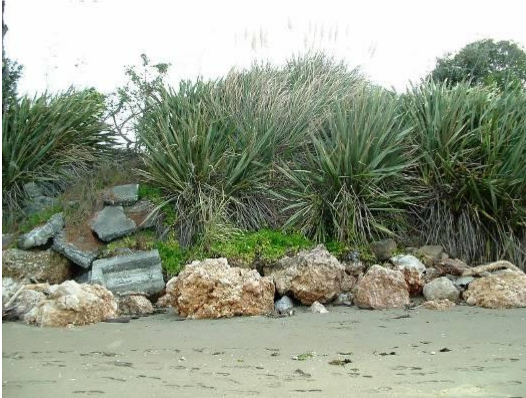
Photograph 5: Photograph illustrating the condition of much of the existing rock revetment
