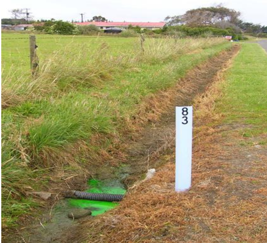
Dye discharge: piped from domestic tank to roadside drain; discharge through culvert onto a Golden Bay beach
