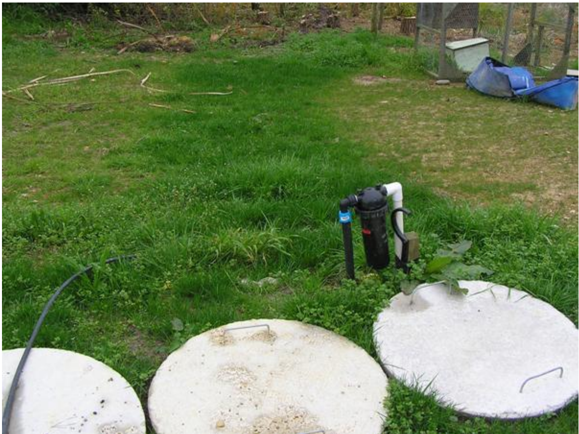
This system services a cluster of 4 old workers accommodation units. Recently refurbished and tenanted full time, the old septic tank system failed to cope with the increased flows. Note: the lush green grass growing where the sewage overflows from the tanks. In this case the flow runs down through the tenant vegetable garden and into an open drain discharging into the Mariri estuary
