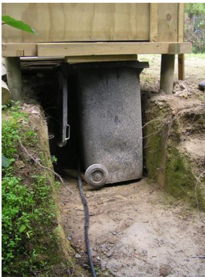
Non complying 'Home made' composting toilet in Moutere area . Bowl sits above the wheely-bin in the cubicle. Urine passes through the black pipe into a dry swale.
