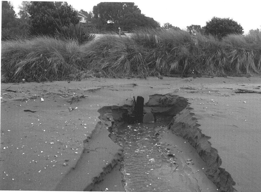
DRAINAGE FLOW NEAR WOMERSLEY'S PROPERTY SEPT 29
