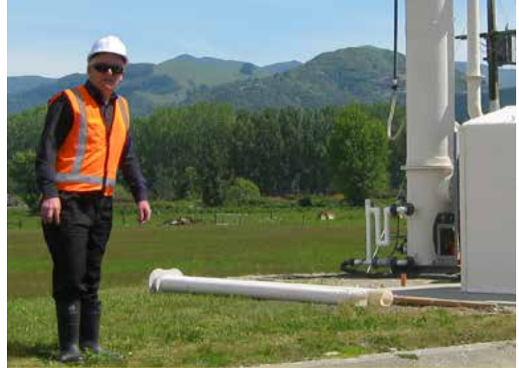
Robert Workman at the Motueka Odour Control Unit
