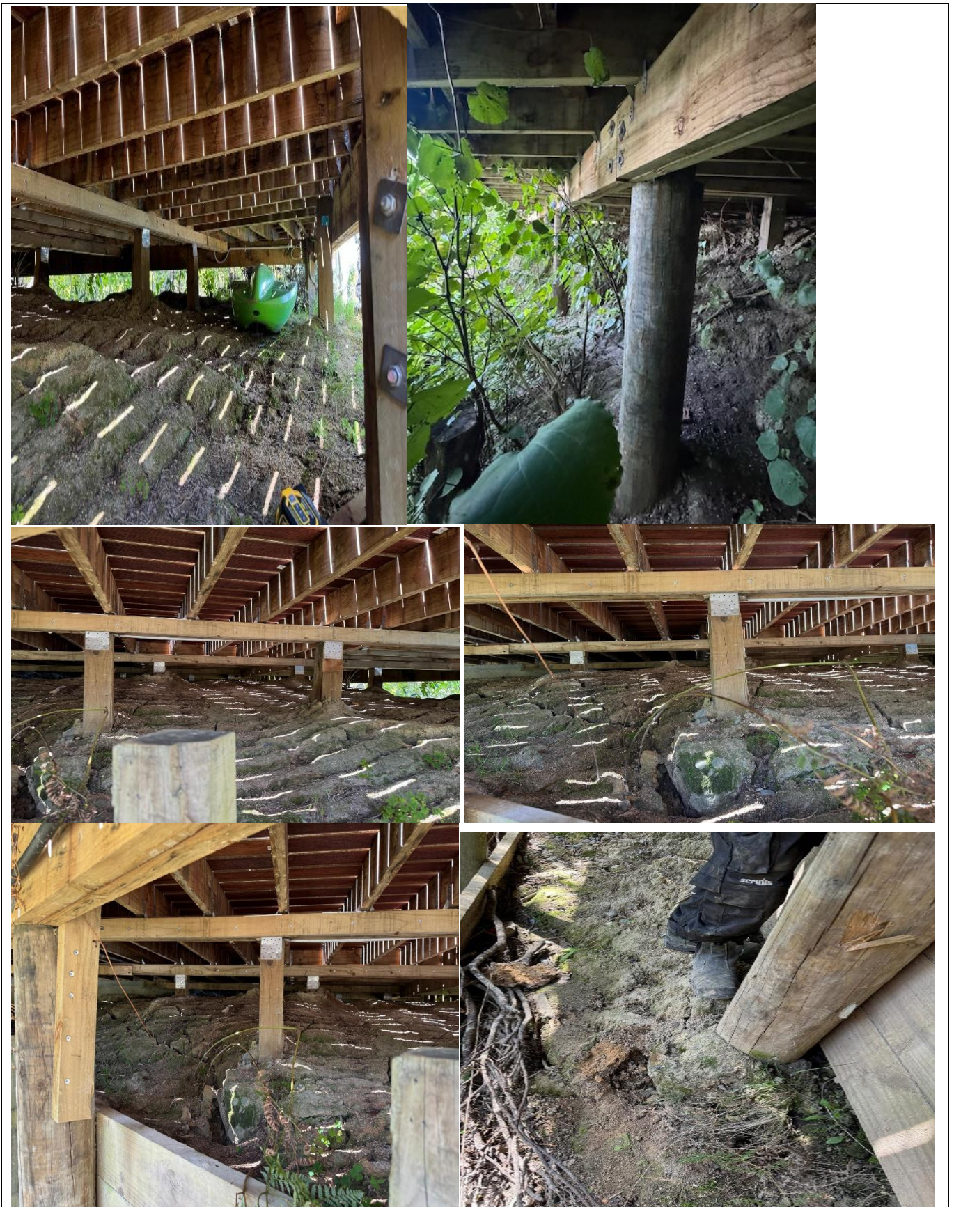
Fig 1- 6 Above, show surfaces that need erosion protection to control upper sandstone instability, which can be achieved using sealed DPM
