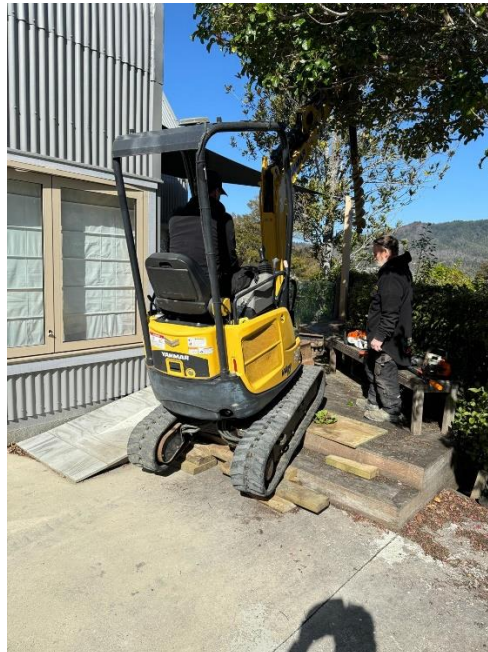
Figure 4. - Excavator positioning on deck for SH2 sample hole with existing dwelling to the left
