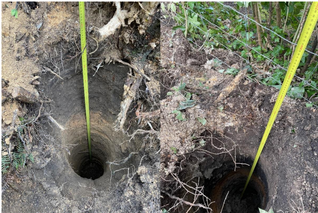
Figure 7b & 7c. – Construction images of the post holes depths. More images are included in the appendix under PS3 images.
