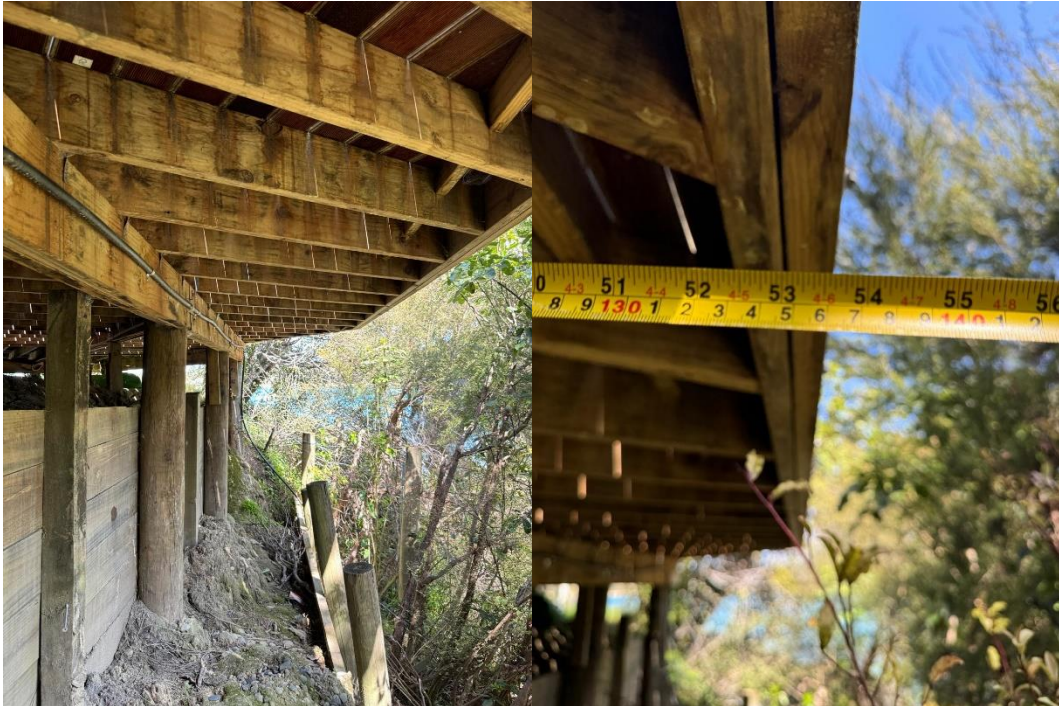
Figure 6a & 6b. - Row of Round Posts with 1m high retaining wall held by square posts (left) and 137cm overhang of deck from row of piles (right) along the west edge of the deck
