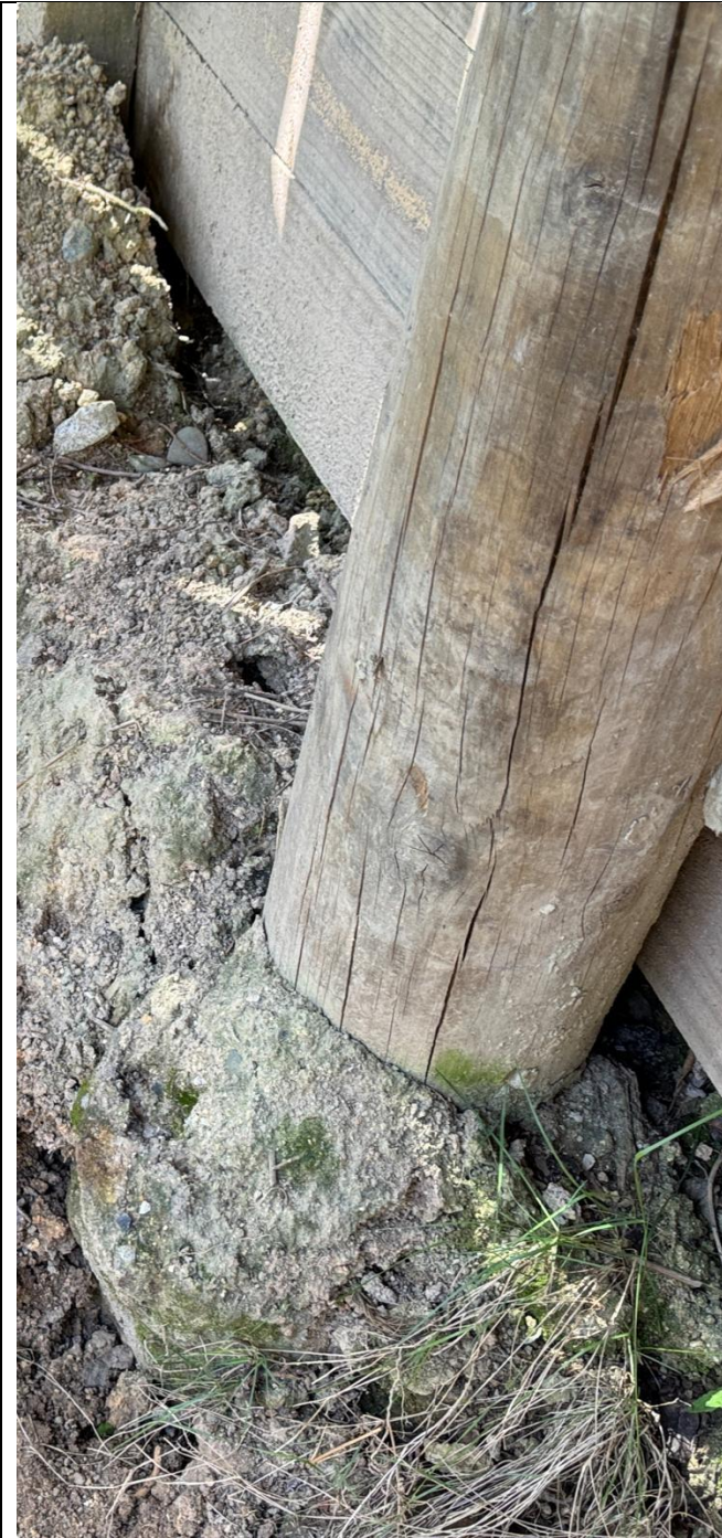
Figure G1. – Post to ground interface that highlights the top of the concrete partially hidden by topsoil used in the soil loading calculations. Additionally, the image shows the importance of placing waterproof membrane around the base of the pile to protection from weathering and erosion.
