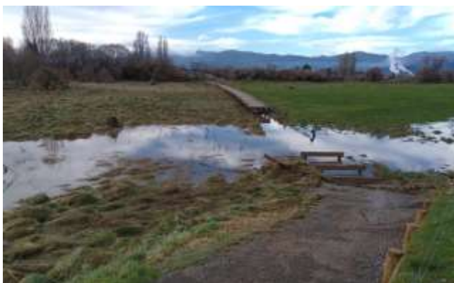
The reserve is vulnerable to flooding. This section of boardwalk on Tasman’s Great Taste Trail (just south of the reserve area) was damaged after the July 2021 flood event.
