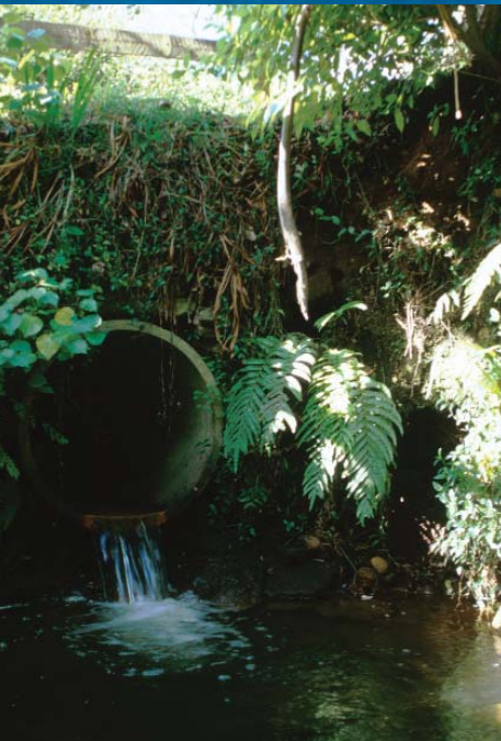
Poorly designed culvert (no level with bed, no fish access)
