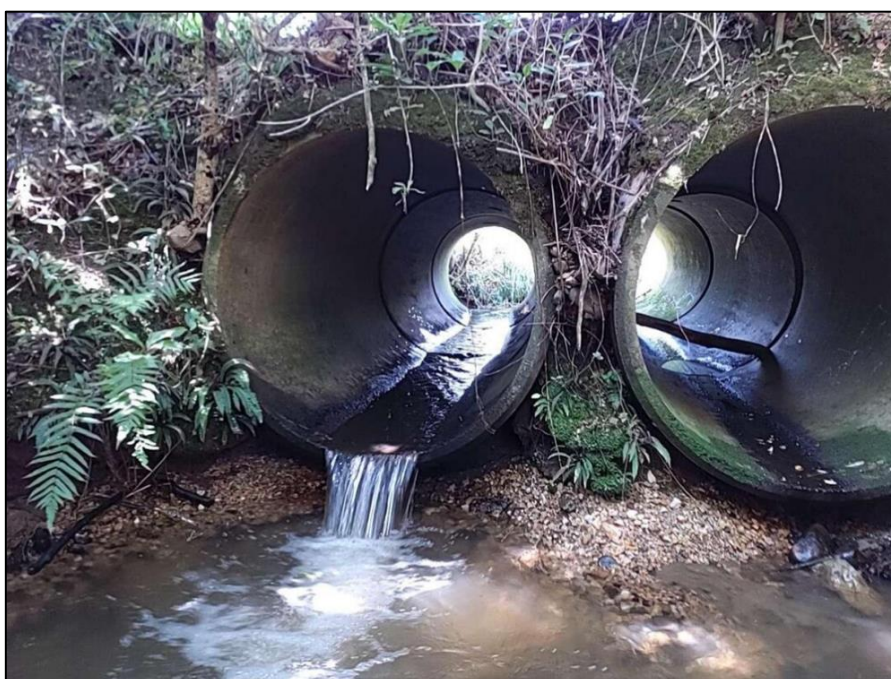
Figure 16. Perched culverts at Mulligans Creek (prior to any remediation for fish passage).
