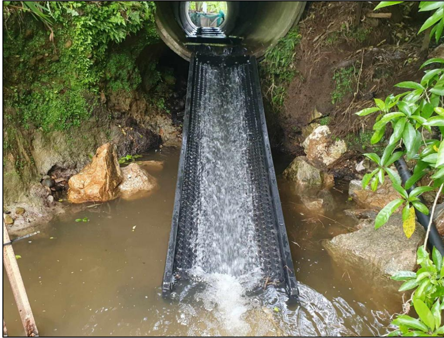
Figure 21. The remediation at Shambhala Creek on the true right culvert, including a floating fish ramp and flexible baffles.
