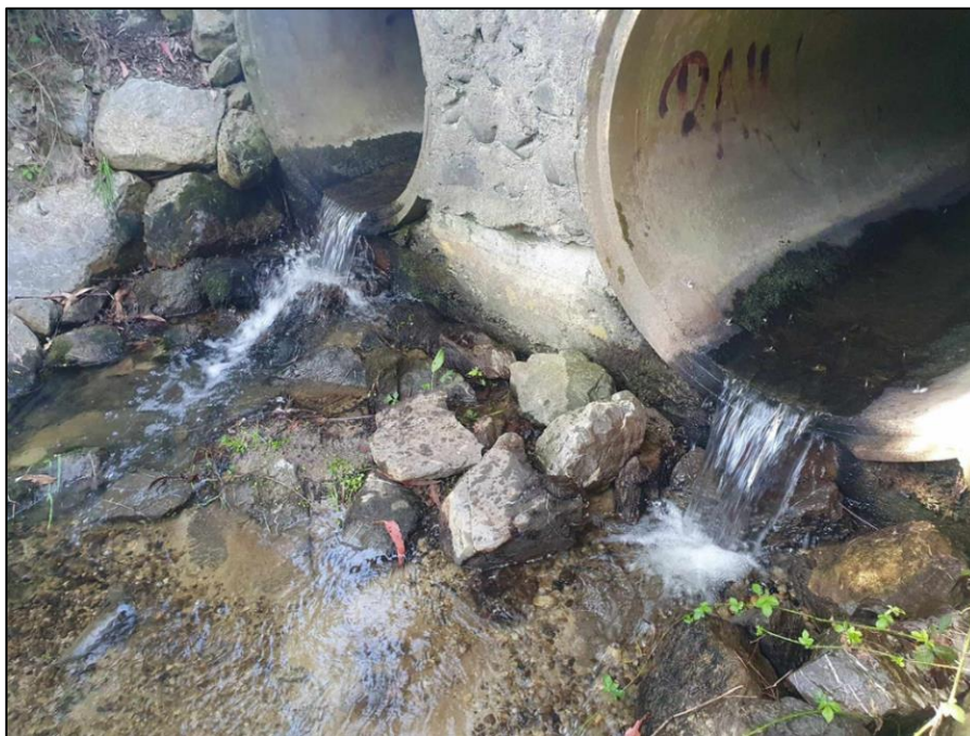
Figure 10. Perched culverts at Williams Creek in September 2023 (prior to any remediation for fish passage).
