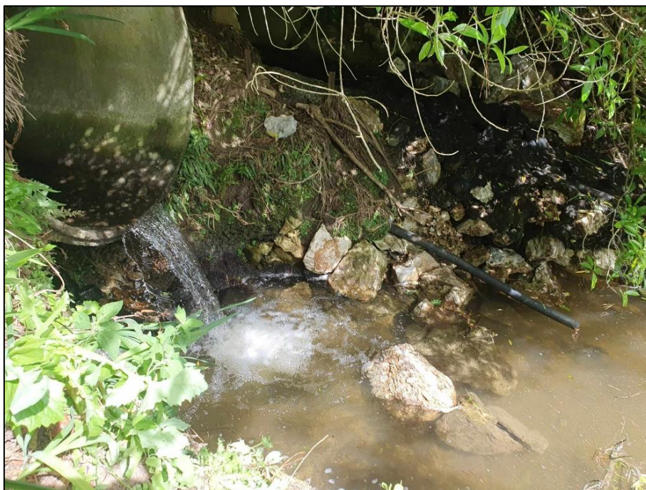
Figure 19. Perched true right culvert at Shambhala Creek (prior to any remediation for fish passage).
