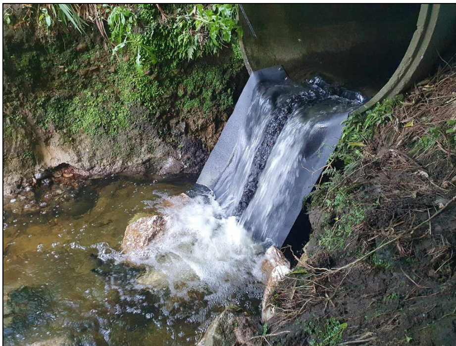
Figure 20. The remediation at Shambhala Creek on the true right culvert, showing a flexible rubber ramp with mussel-rope and a V-baffle.
