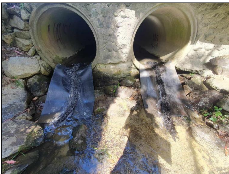
Figure 11. The remediation at the Williams Creek culverts, showing two flexible rubber ramps with mussel-rope and V-baffles.
