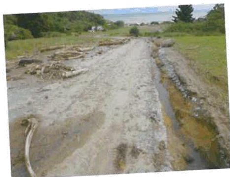
Photograph 4-4: Damage to the Matenga Road carriageway, evidence of the carriageway acting as a major overland flowpath during this event.
