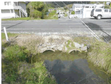
Photograph 7-8: Twin 1200 mm diameter culverts under Abel Tasman Drive downstream of site (looking upstream). Water level controlled by downstream dunes; photo taken at low tide.
