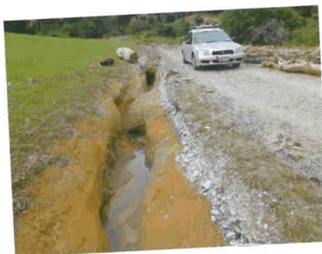
Photograph 4-5: Scour in excess of 1 m depth in roadside drains along Matenga Road.
