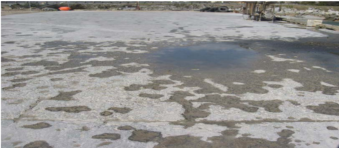
Photograph 2: Abrasion to wharf surface caused by placing/ moving rock or mussel anchor blocks on wharf.
