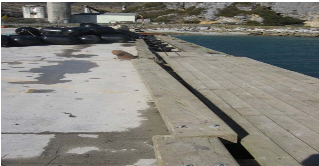
Photograph 3: Loose timber kerb at edge of wharf.
