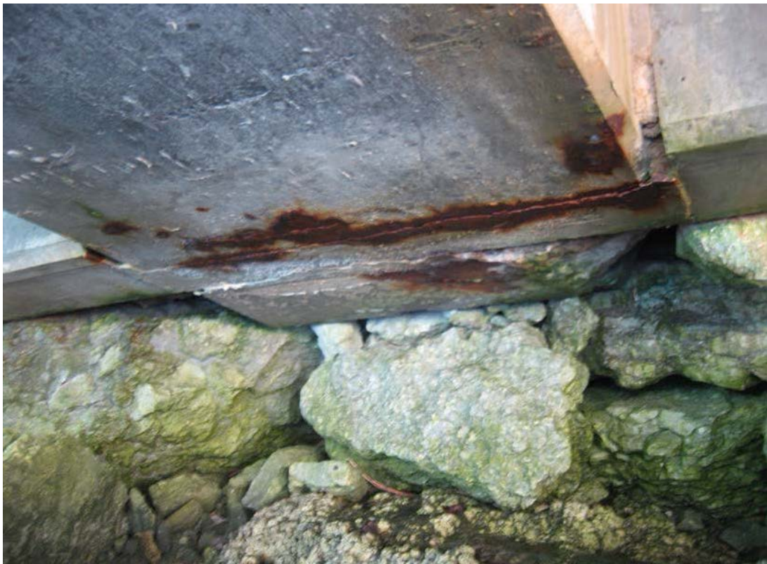
Photograph 9: Typical cracking and rust staining to underside of beam joint on landward side of wharf.
