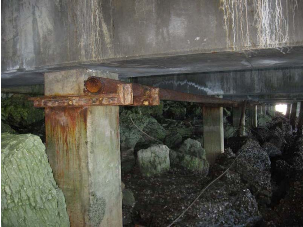
Photograph 10: Disused pipework and steel supports causing rust staining to concrete piles.
