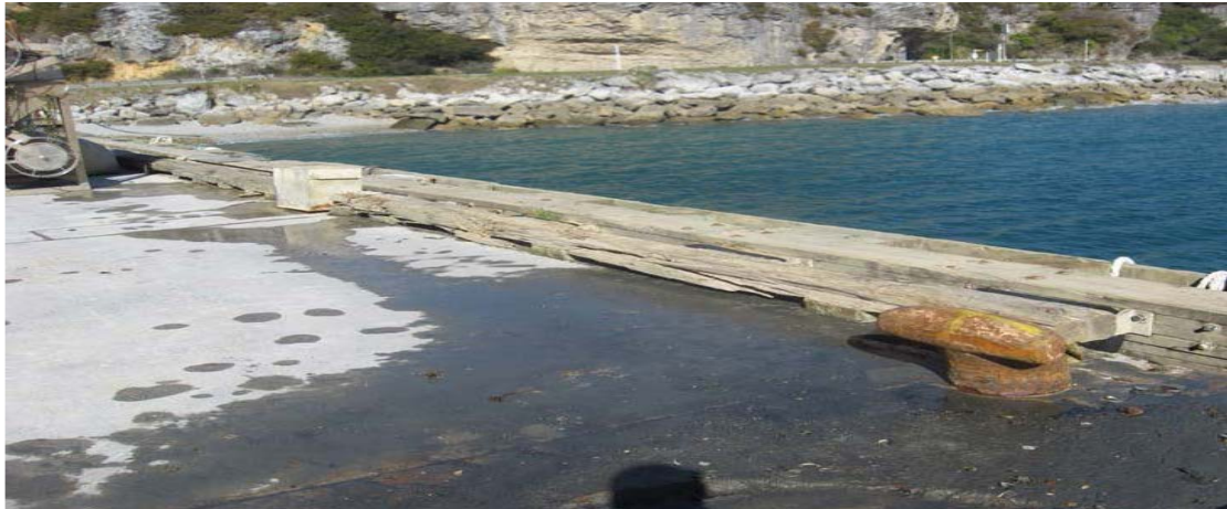
Photograph 4: Damaged timber kerbs.
