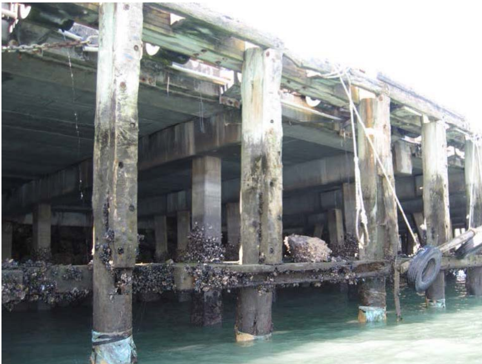
Photograph 11: Showing large section loss in horizontal timber member of fender system.
