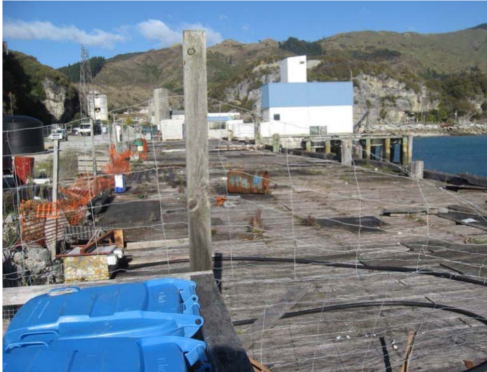
Photograph14: View of deck of timber wharf (condemned and retained for future development).
