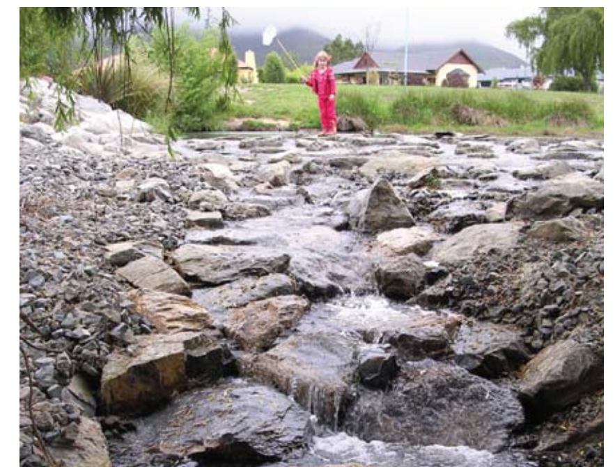
Fish passes like this rock ramp in Reservoir Creek below Templemore Pond (Richmond) help native freshwater fish swim upstream past perched obstacles.
