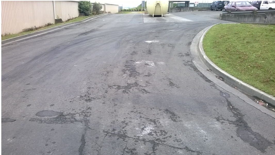
Figure I-4: Example of Aged Chip Seal Suffering from Scabbing and Cracking
