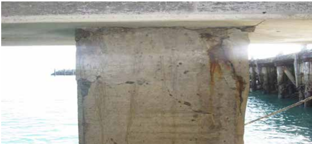
Photograph 6: Typical spalling of concrete at top of piles.
