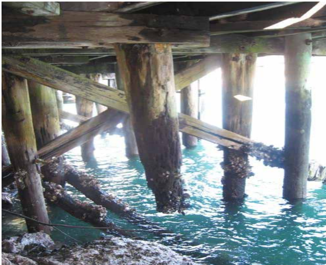
Photograph 15: Showing badly deteriorated pile that no longer reaches the water.
