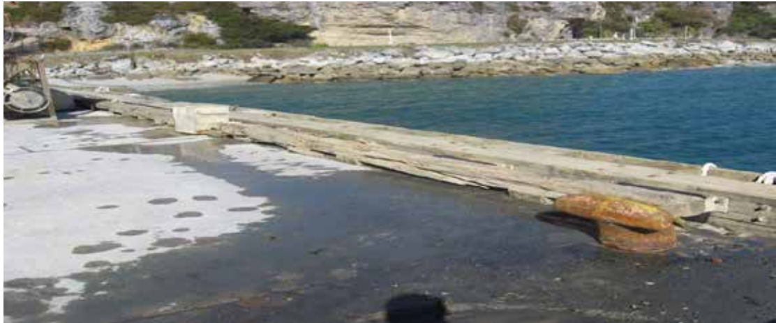
Photograph 4: Damaged timber kerbs.
