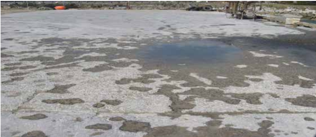
Photograph 2: Abrasion to wharf surface caused by placing/ moving rock or mussel anchor blocks on wharf.
