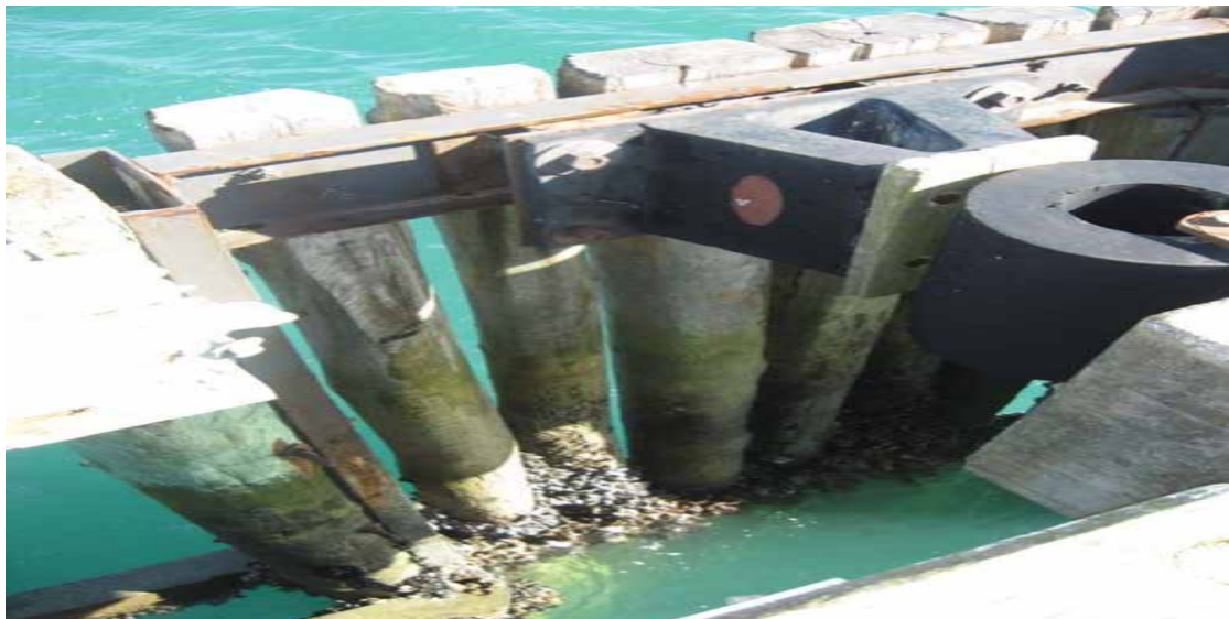
Photograph 5: Showing rubber components of fendered system.
