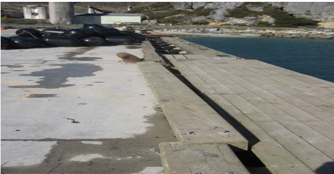
Photograph 3: Loose timber kerb at edge of wharf.
