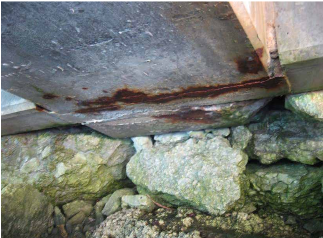
Photograph 9: Typical cracking and rust staining to underside of beam joint on landward side of wharf.
