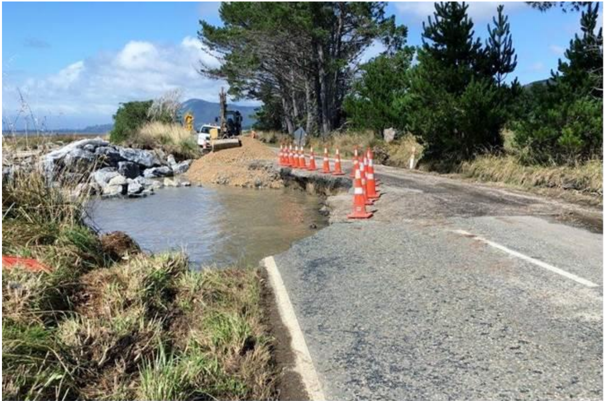
Washout on Collingwood-Puoponga Main Rd
