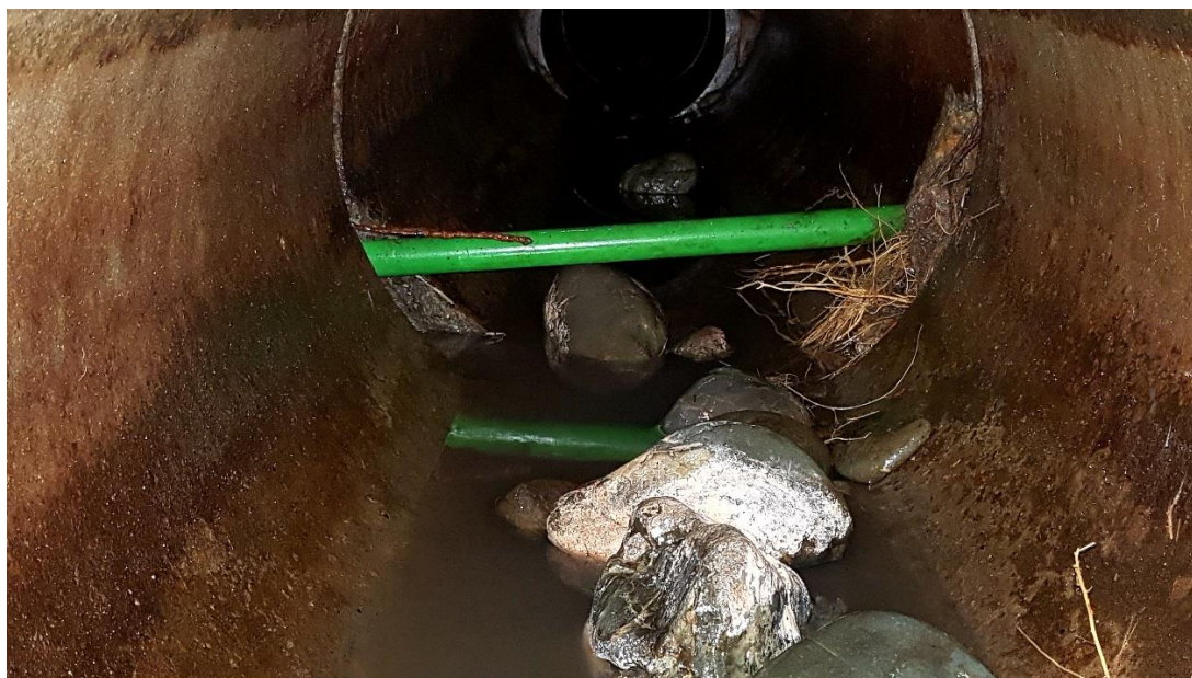
UFB duct through stormwater pipe Elizabeth Street
