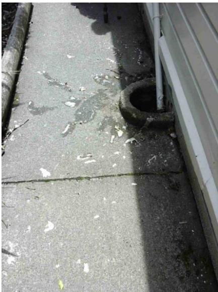
Mapua School Overflow - 17 January
