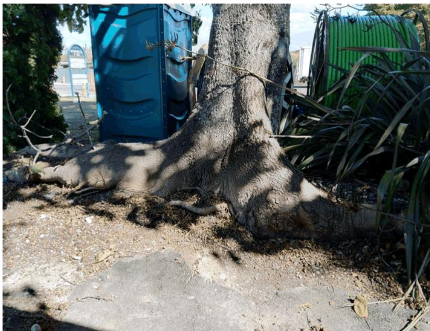
Photo 2: showing root system of tree constrained within old narrow planting strip. Some damage to the hard surfacing can be seen in the foreground.
