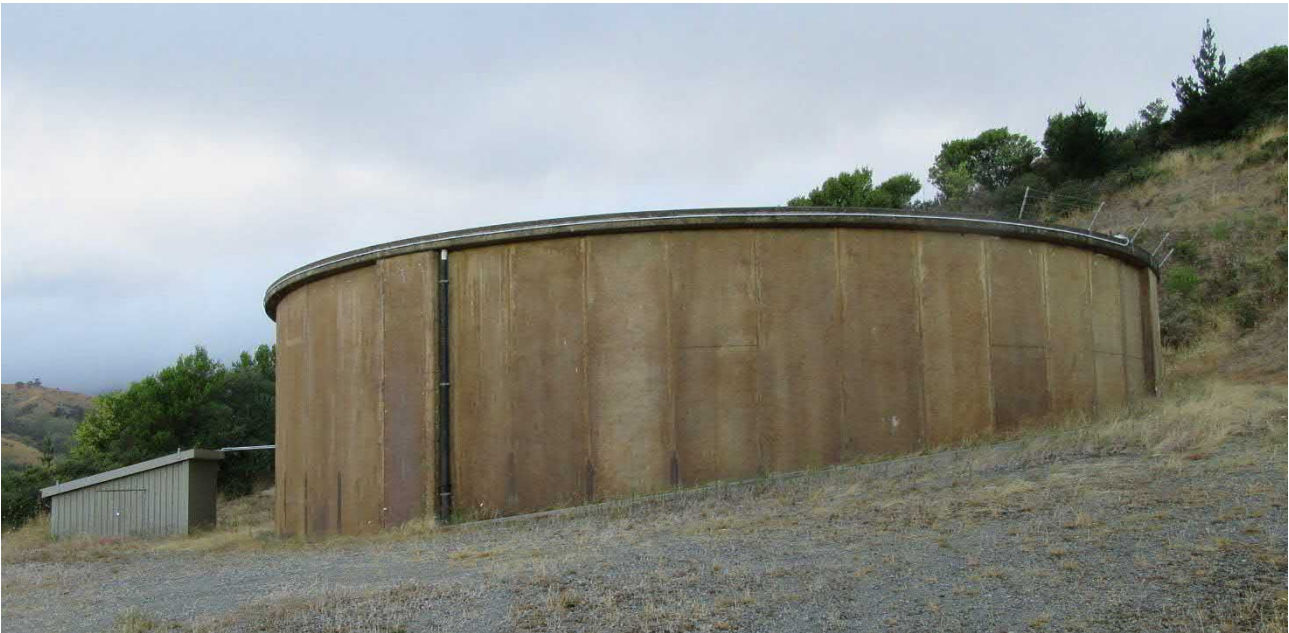
Figure 4 Existing water tank at Marsden Valley, Stoke, Nelson with 'Permeon' colouration/oxidation process applied to the raw concrete ( Photograph taken 3 February 2020, by Noelia O'Leary, design engineer, WSP ).
