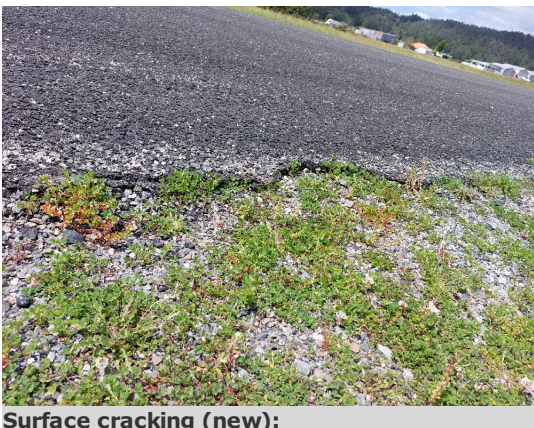
Surface cracking (new):
