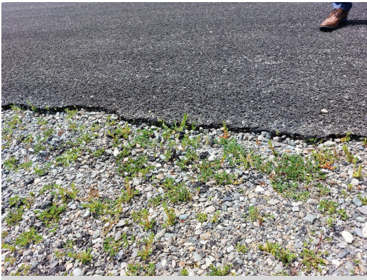
Surface cracking (new):
