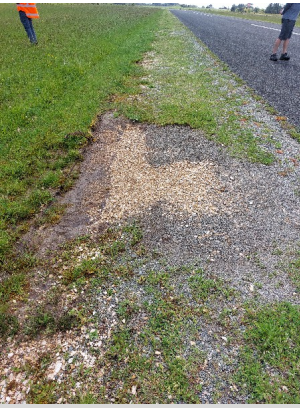
Hazardous ruts, humps, depressions, unusual surfaces:
