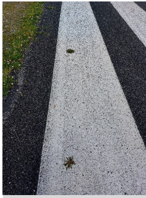
Surface cracking (new):
