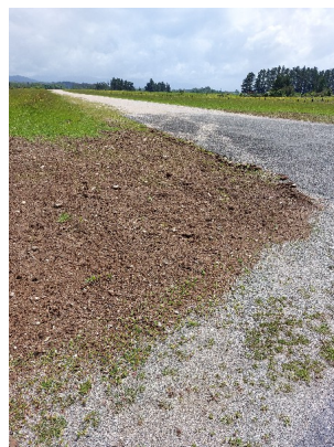
Hazardous ruts, humps, depressions, unusual surfaces:
