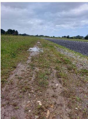
Hazardous ruts, humps, depressions, unusual surfaces:
