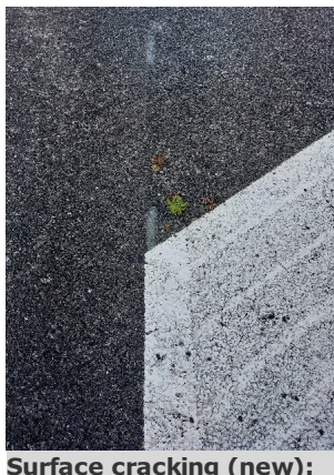
Surface cracking (new):
