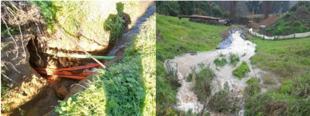
Exposed services (L), temporary diversion of watercourse away from services trench (R) - Pohutukawa Place, Pohara.
