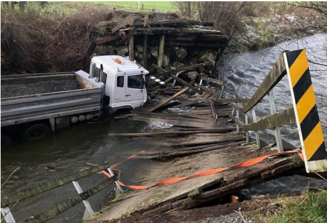
Creighton Road Bridge damage
