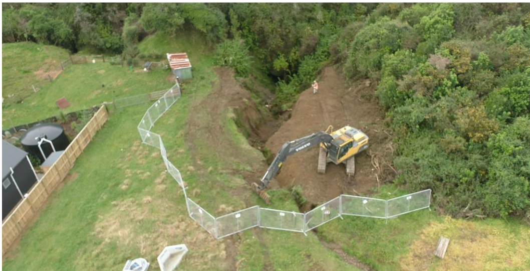
Open channel erosion in Pohutukawa Place, Pohara. Exposed services in foreground, adjacent to fencing, outlet tomo in the background.
