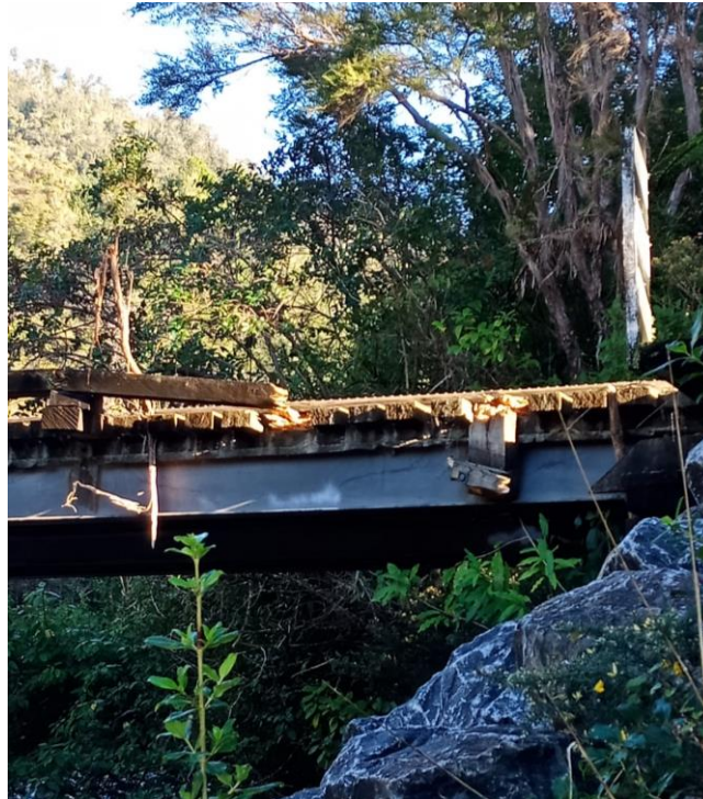
Walsh Creek bridge damage
