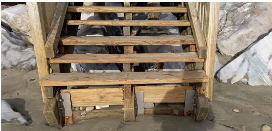
Old Mill Walkway showing degrading of foreshore April 2021
