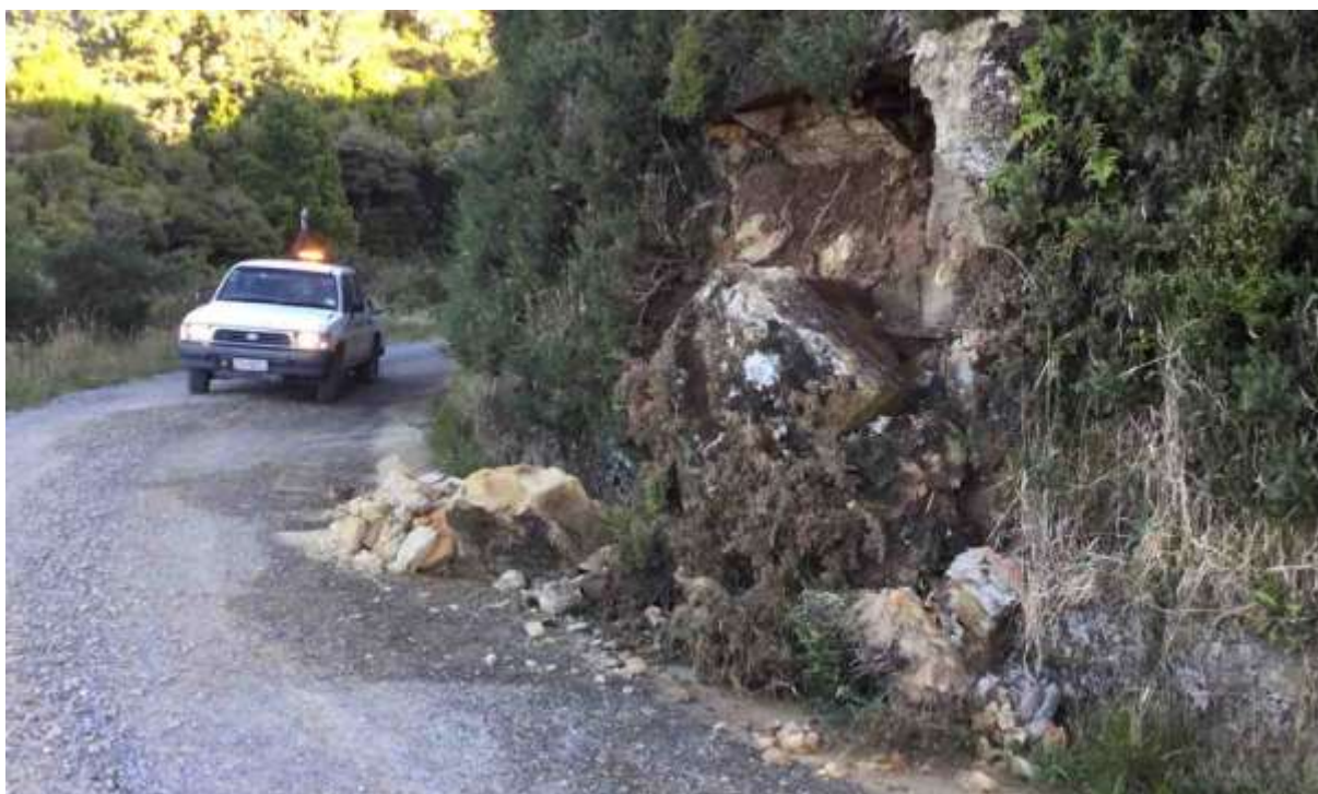
Te Hapu Road slip
