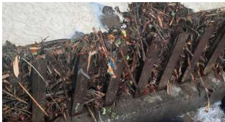
Normal hillside debris collected on grills at stormwater pipe inlet Easby Park, Richmond on 2 March
