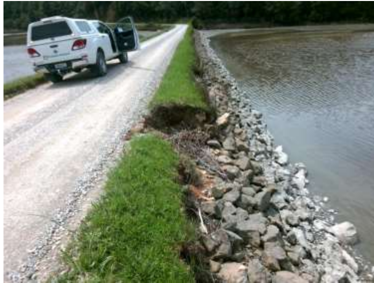
Dry Road protection damage
