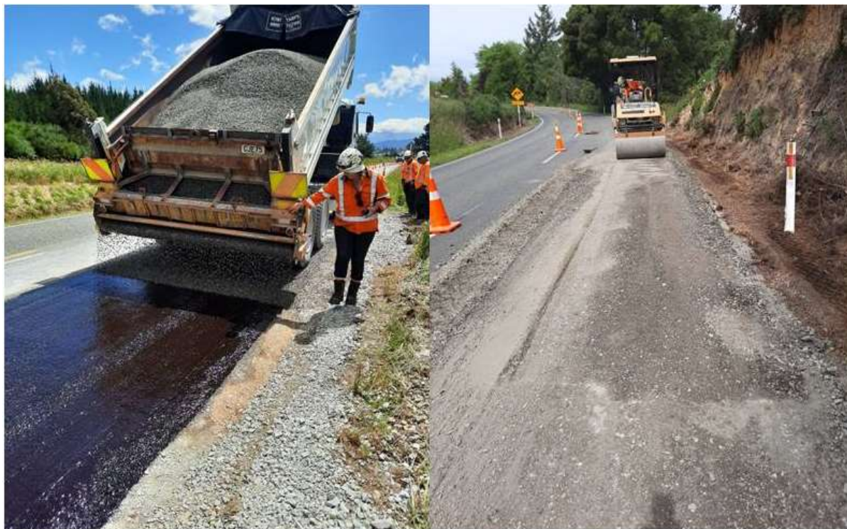
Left: Emulsion Stabilising sealing Right: Emulsion Stabilising compacting stabilised material – Moutere Highway
