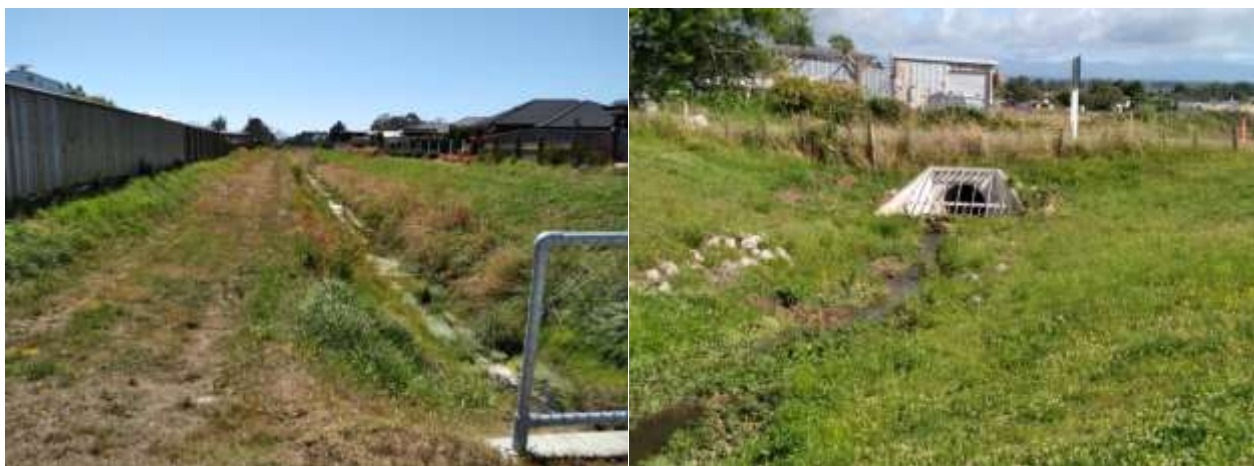
Typical ongoing growth of open drain banks at Morley Creek, Iwa Street, Mapua (L) and Bateup Creek, Paton Road, Richmond (R)
