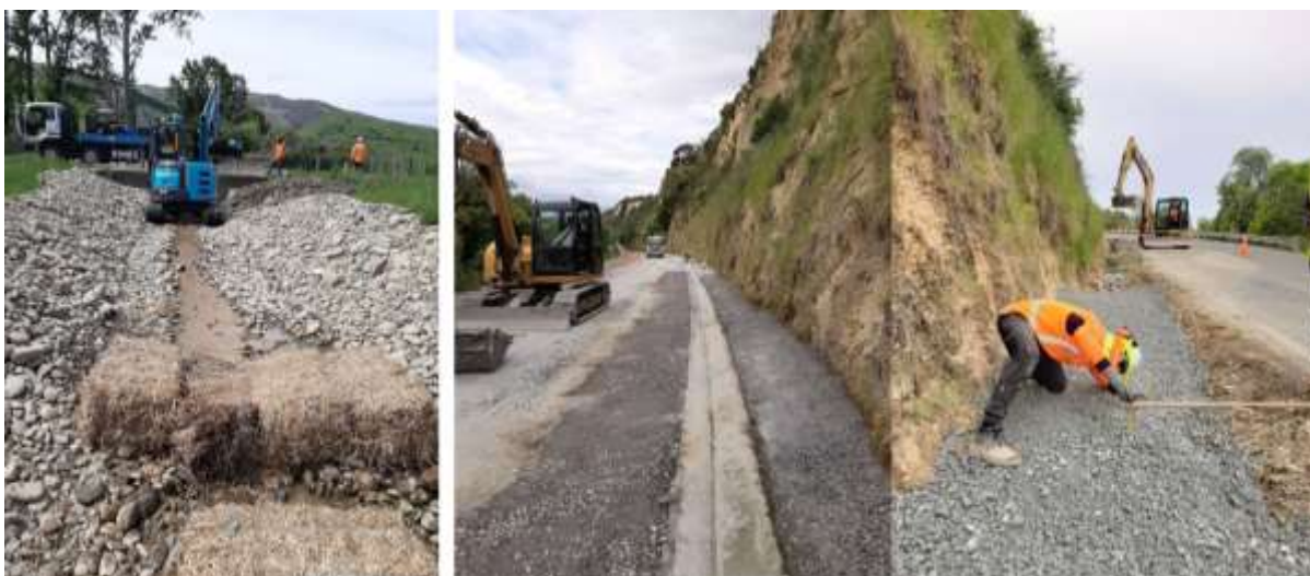
Left: Tadmor Valley culvert clearing, Middle and Right: MBIE Stafford Drive under slip remediation
