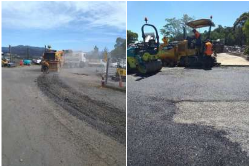
Milling of pavement (L) and placement of new pavement (R) at the Māiri Resource Recovery Centre
