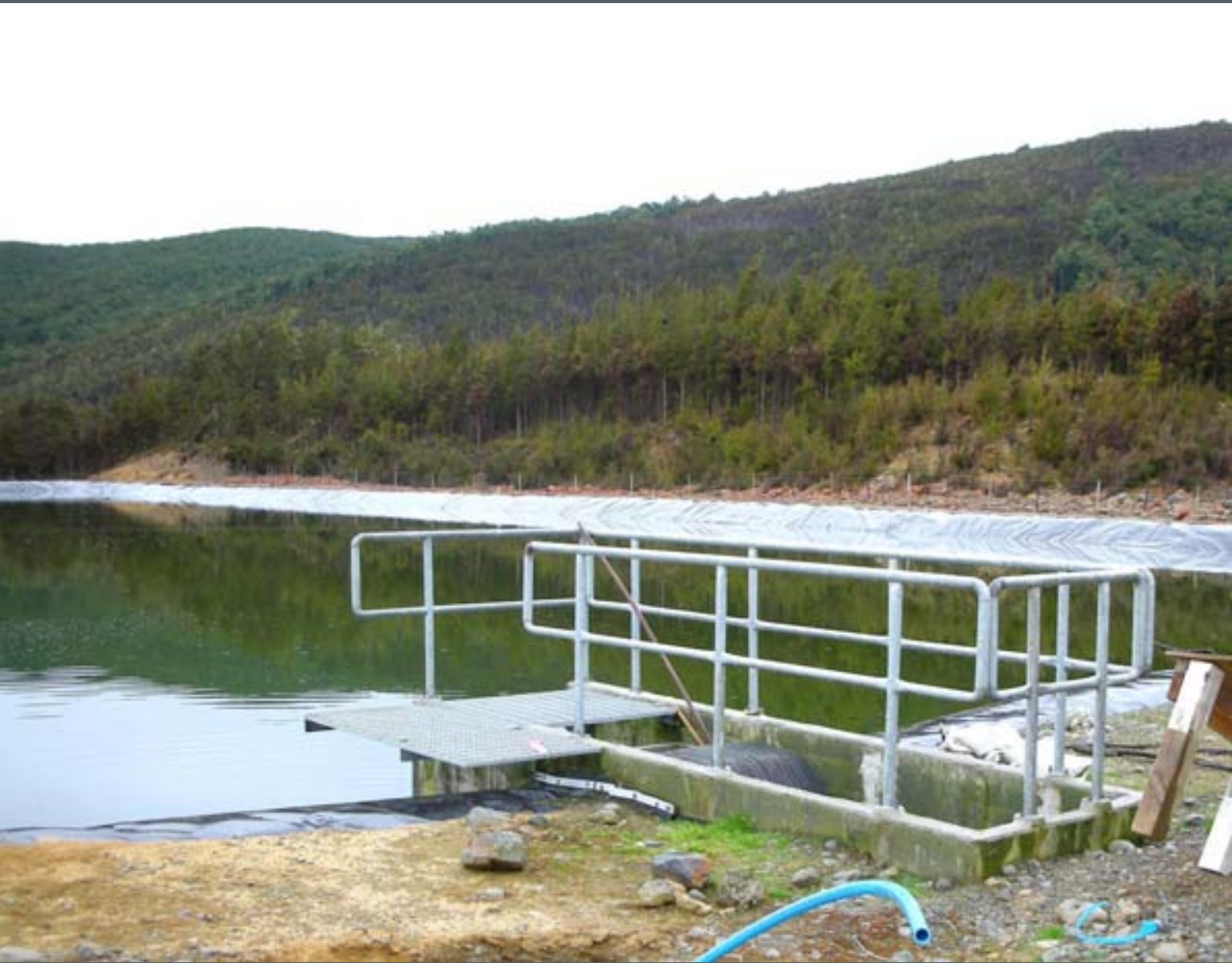
St Arnaud wastewater treatment plant.
