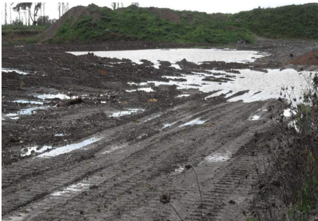
Figure 21. Spreading compaction and drainage impairment.
