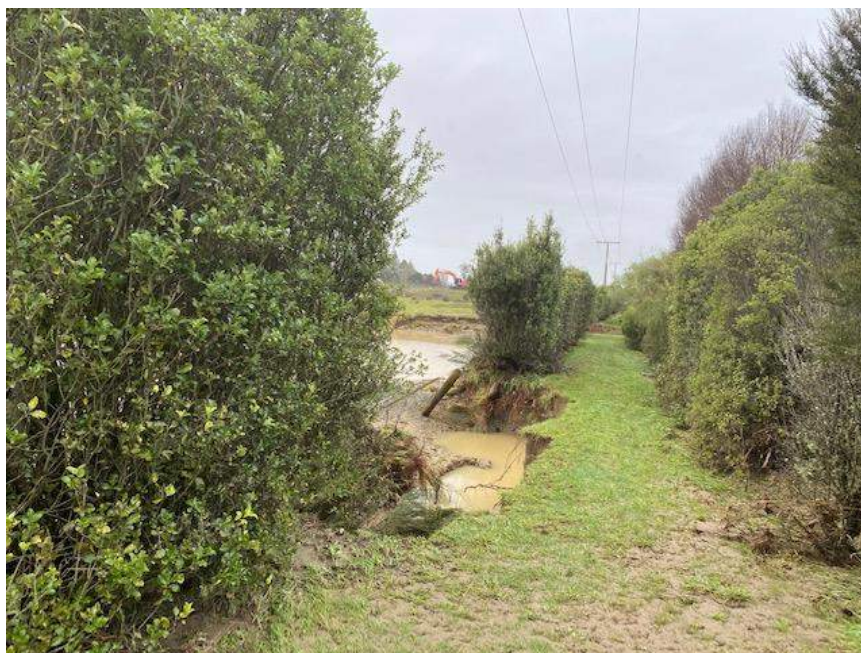
Figure 7. View east of the headcut erosion of fine-grained sediments at the upstream end of the northern pit at Douglas Road following the 17-18 July 2021 flood (Photo provided by Pete Taia)
