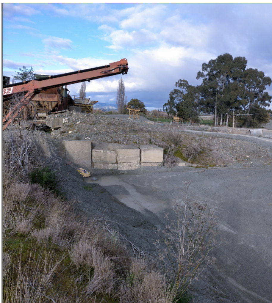
Figure 6 – The portion of compromised stop bank to be realigned
